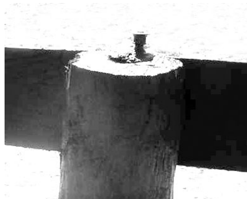
Figure 3. Treated pine post. The sapwood was properly preserved, but the untreated heartwood began to rot underneath the paint. Brush-on remedial preservative treatment would probably have helped this particular post.
