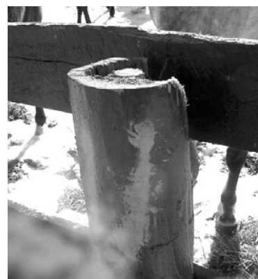
Figure 4. Treated pine post. Untreated wood began to rot, with the sapwood being more significantly affected than the slightly more rot-resistant heartwood. This degree of sapwood degrade would not be expected for properly preserved wood, so this particular post may have had an inadequate preservative treatment. Its poor condition was probably worsened by the lack of after-cutting preservative treatment and by the paint applied soon after installation that trapped water within the post.
